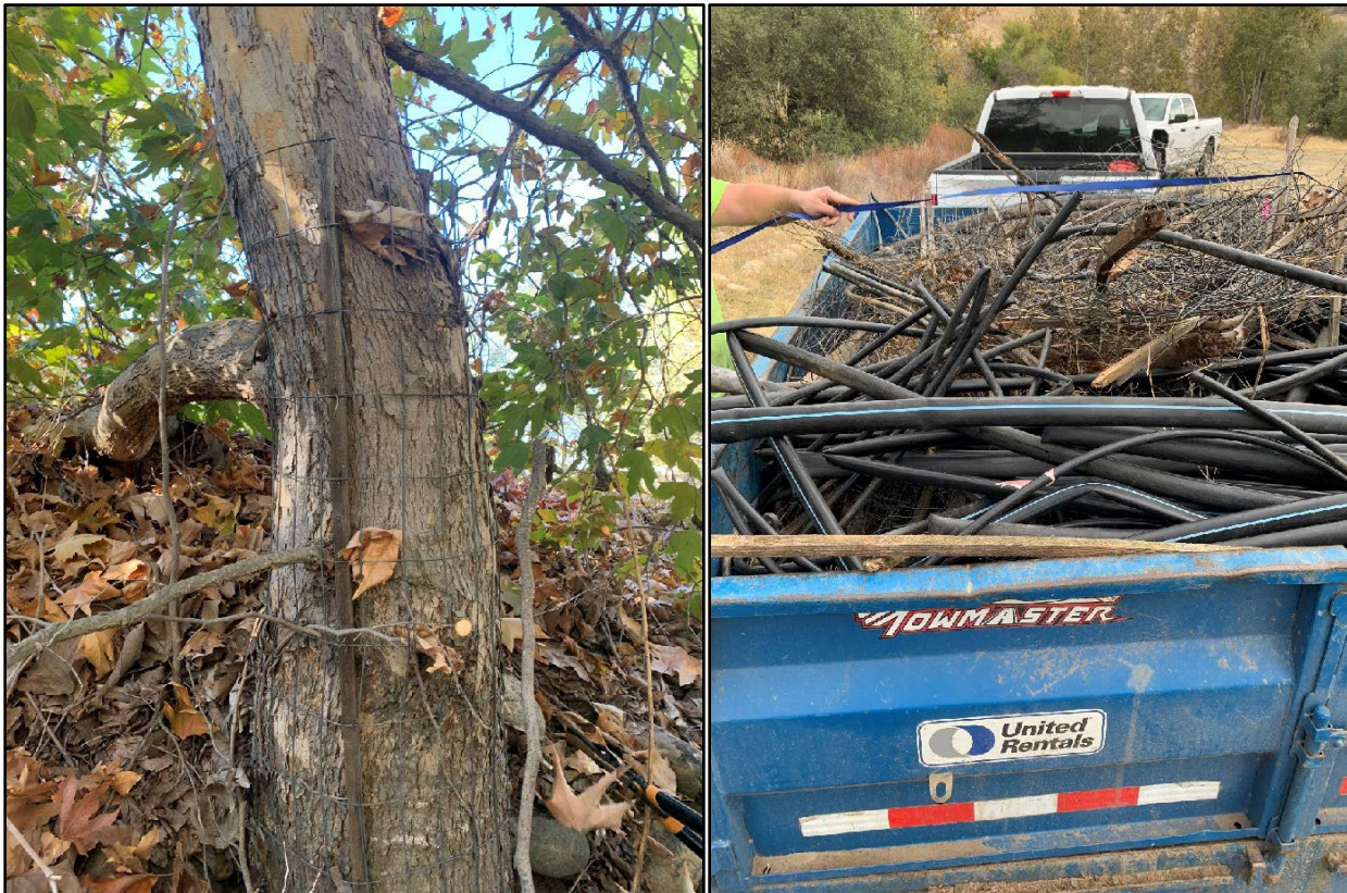
Figure 8-1: On left, tree growing inside wire cage prior to cage removal, and on right, trailer load of removed tree cages and drip irrigation line from the Thorburn Channel.
