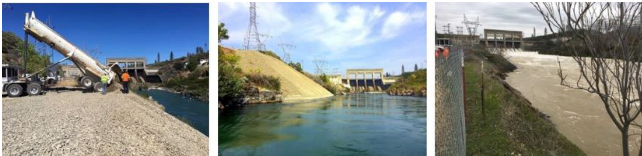
Figure 46. Bankside gravel injection is one of the older methods of adding gravel to sediment starved rivers to improve spawning habitat. Photographs courtesy of J. Hannon (USBOR). This process relies on the river's energy to mobilize and distributed coarse sediment. Note gravel "dump" during low flow period (left), gravel stockpile (middle), and gravel mobilization during high flow period (right).
